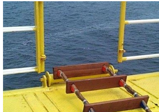
Figure 1: Handholds that terminate above the vessel structure.
